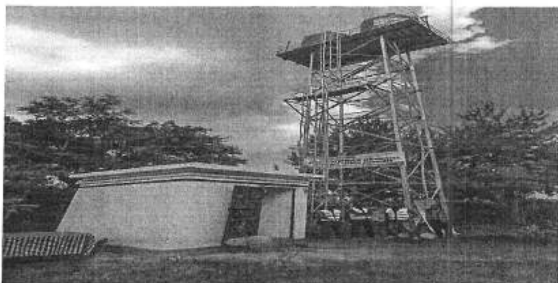
Solarization of Gathanji borehole in Githunguri sub County
