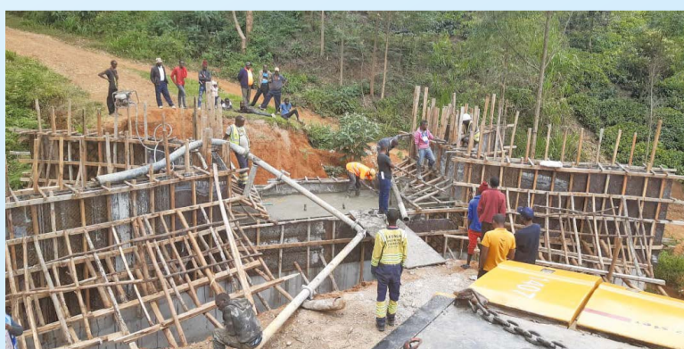
Mariguiti Bridge in Kiganjo Ward Gatundu South is almost complete with concreting of deck now complete.
