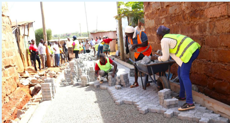
Construction of link cabro roads in umoja informal settlement within Thika Municipality.
