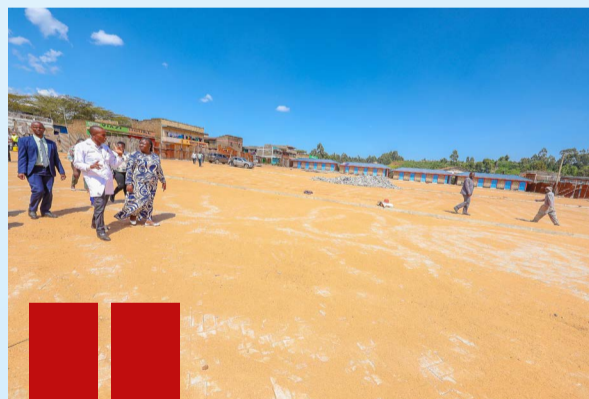
Kiambu Governor Dr. Kimani Wamatangi inspects the ongoing Kwambira Bus Park project in Limuru Township, Limuru Sub-County.
