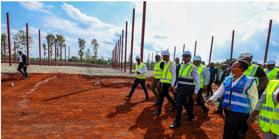
Ongoing County Aggregation and Industrial Part at Warugiu in Ngewa, Githunguri Sub-County.
