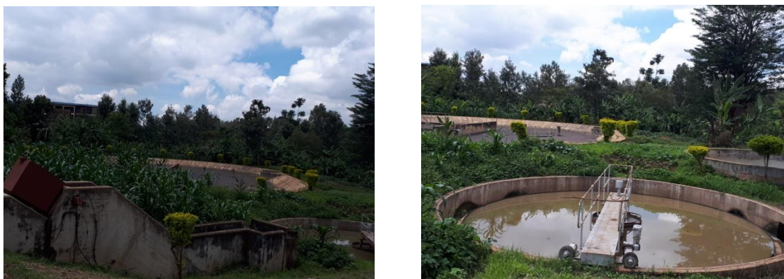
Figure 4: Limuru Sewerage Treatment Works
