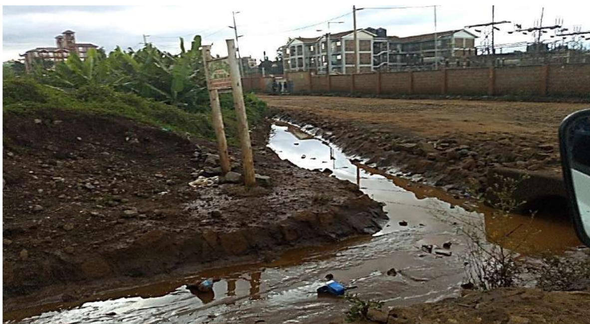
Figure 8-11: A Stormwater Drain in Gachie Urban Centre
