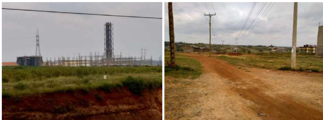
Figure 8-14: Power Sub Station and Electricity Distribution Lines at Witeithie
