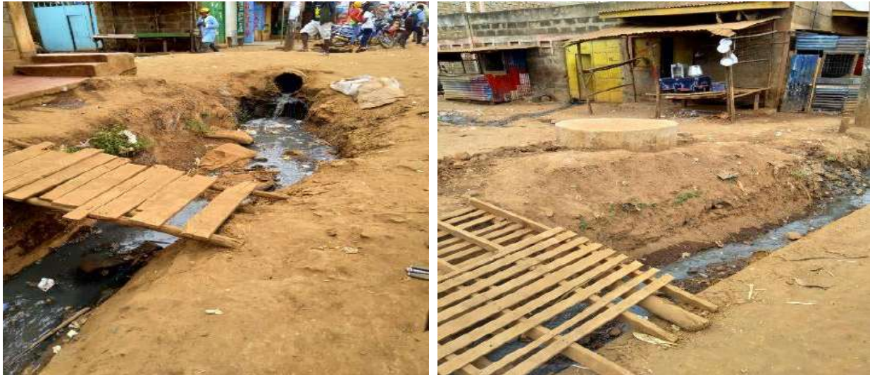
Figure 8-12: Poor stormwater drainage systems in Witeithie
