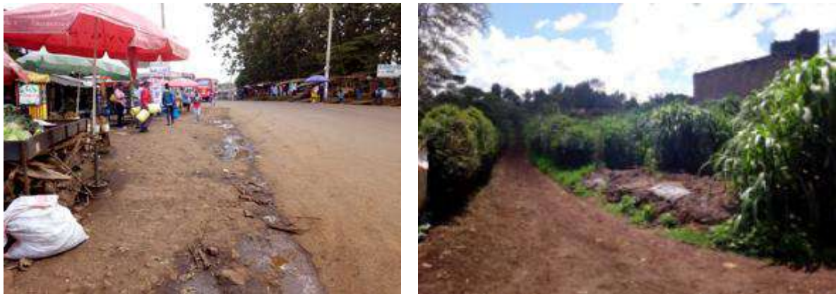
Figure 10: Road condition in Kiambu town
