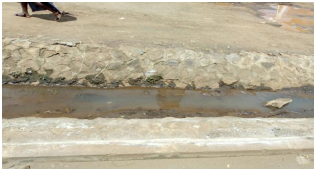
Figure 1: Storm Water Drainage in Kiambu Municipality
