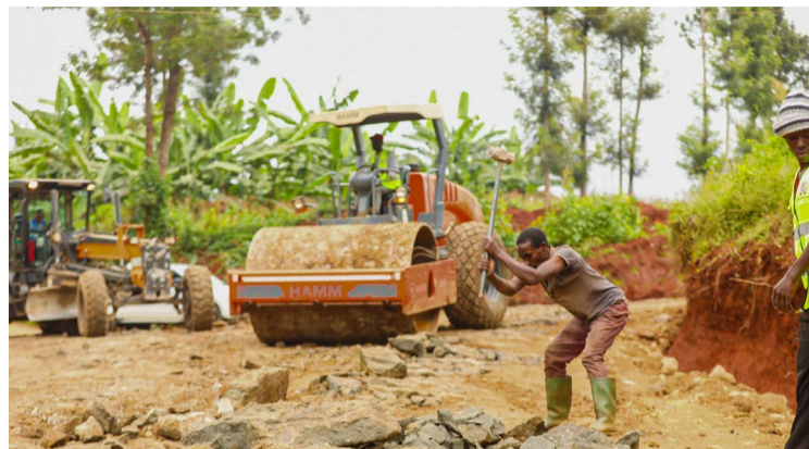
Ongoing construction of Ha-Mwenjera- Muthandi Primary School- Kambi ya Ihi access Road in Kamburu Ward, Lari Sub-county.
