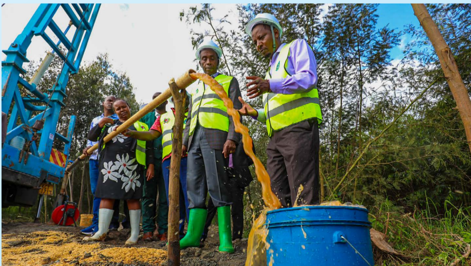
Inspection of the ongoing Makutano Primary School Community borehole Project in Ndeiya Ward, Limuru Sub-County
