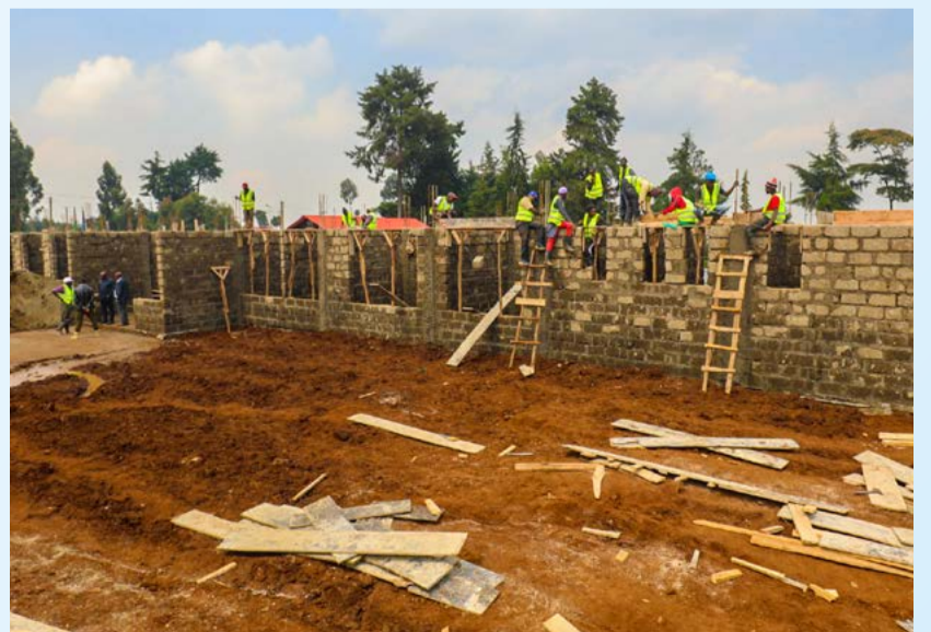
Ongoing works at Kiwaroga Level Three Hospital in Limuru East, Limuru Sub-county.
