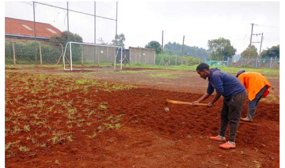
Ongoing planting of grass at Kagwe Stadium in Nyanduma Ward, Lari Sub-County.
