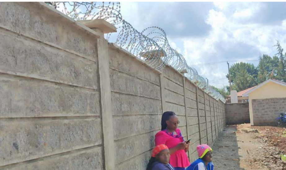
Ongoing fencing of Githunguri Stadium by the Department of Youth Affairs and Sports.
