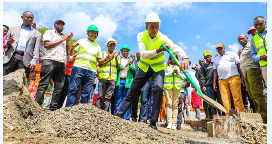
Inspection of the ongoing construction of Lusigetti Market in Nachu Ward, Kikuyu Sub-County.
